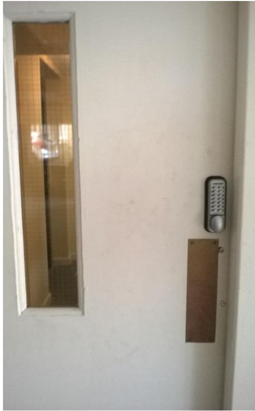
Access to stair well from garage, Repaired painted with new security locks – both doors
